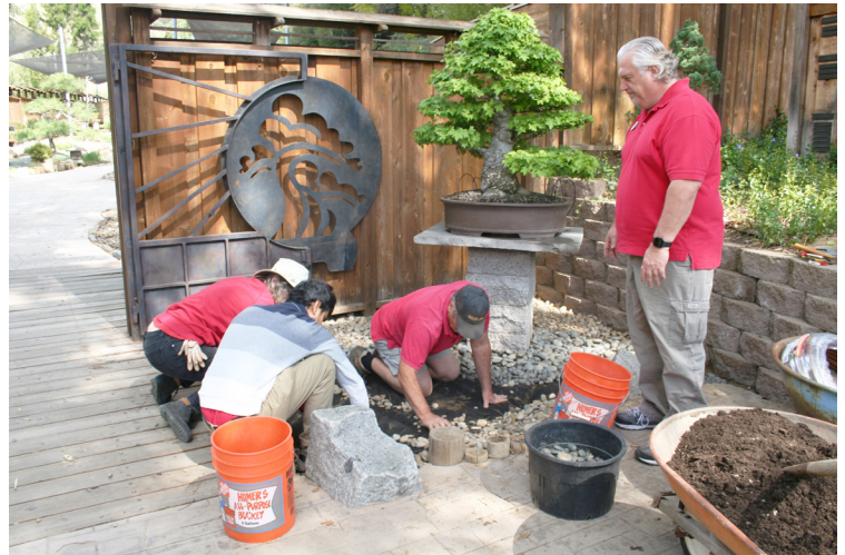
Black weed cloth was put down and the rocks put back in a natural way. The black area will be filled in with Dymondia silver carpet ( Dymondia margaretae ), a hardy, tight growing ground cover with a small yellow flower.
